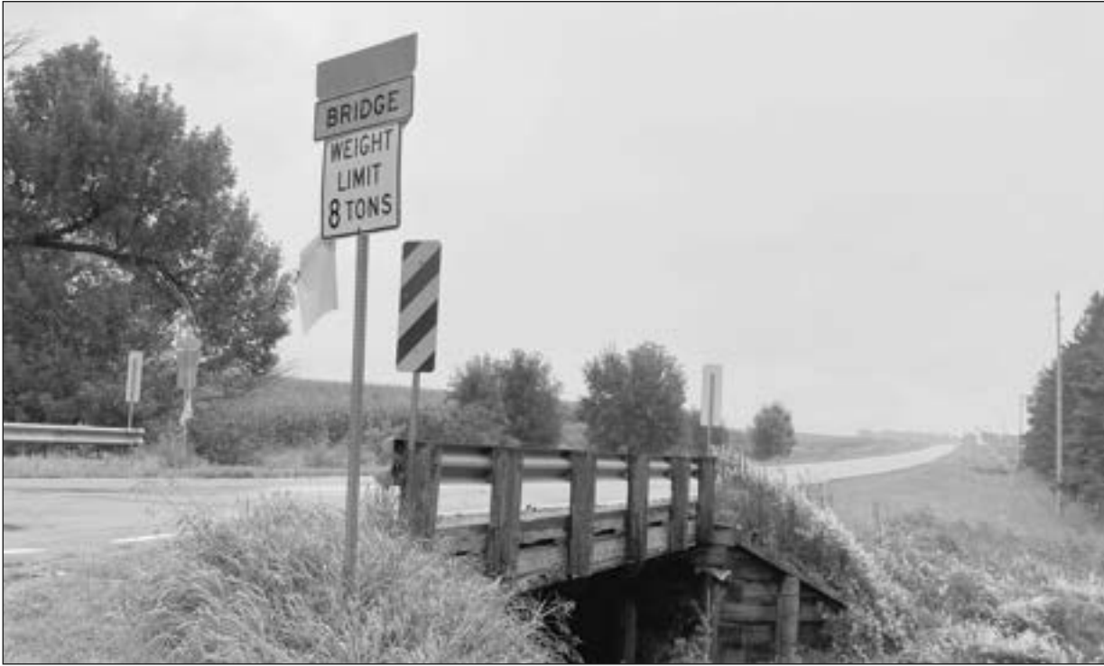
STRUCTURAL CONCERNS- This bridge along County Road 6 northeast of New Richland was built in 1940. Stress tests showed it is no longer safe for vehicles over eight tons. Originally scheduled for replacement in 2027, it will now be replaced in the next few months.
