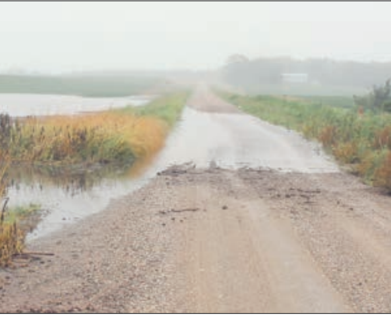
FLOODING - Heavy rains have caused the overflowing of roadways in Waseca County at least twice this summer. Here, rising waters from the nearby LeSueur River caused water to cross a Wilton Township road on July 23.
