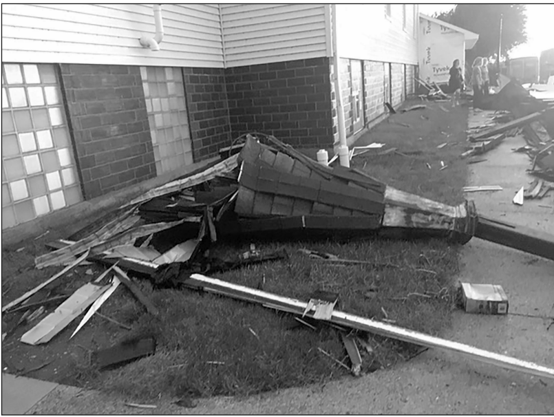
The bell tower and steeple of LeSueur River Lutheran Church, located northeast of New Richland, were broken loose by a tornado in June of 2020 and dropped to the ground nearby. The remainder of the building was relatively untouched. The church was originally built in 1875.
