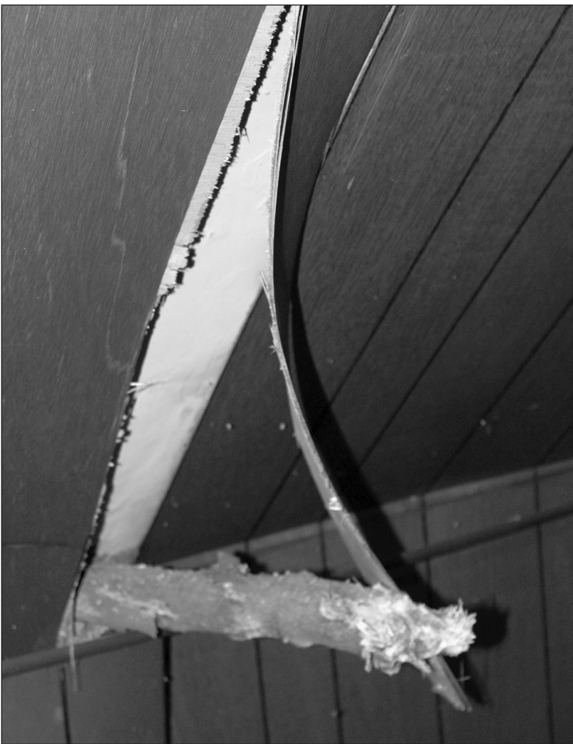
This tree branch, roughly four inches in diameter, punctured the roof of Pam Lab's home located along Highway 30.
